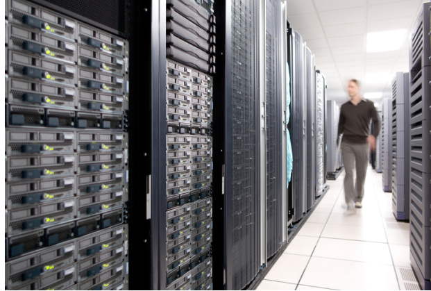
Fig. 1.1 Cisco data center [2].
